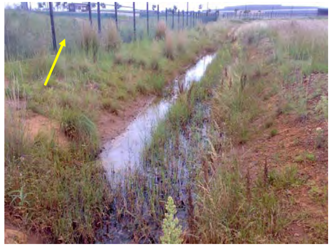
Bio-swale showing good establishment of the wetland grasses and sedges and the new clear-vu fence (2012)
