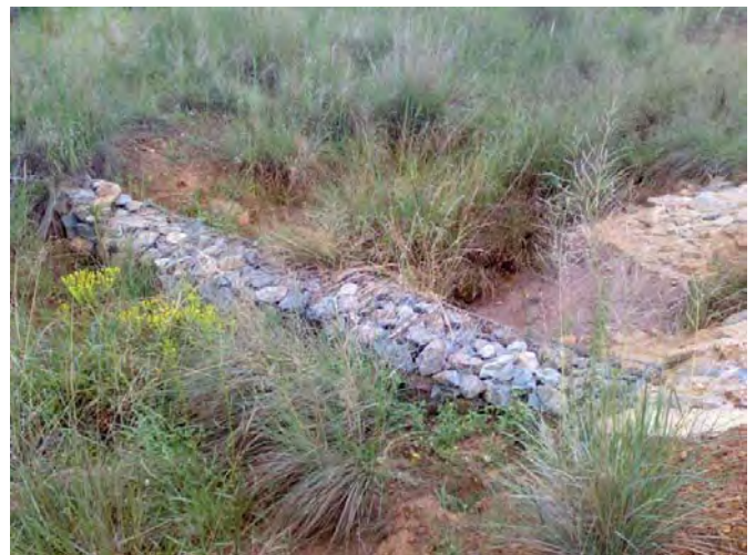
Regrowth of vegetation around the gabions within the bio-swale. The vegetation has re-established well (2012)
