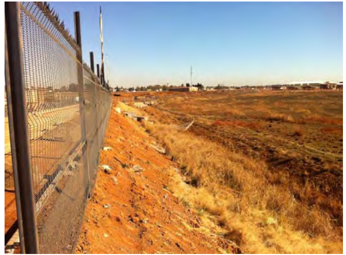
Embankment prior to erosion control measures and hydro-seeding required after new Clear-vu fence installed (2011).
