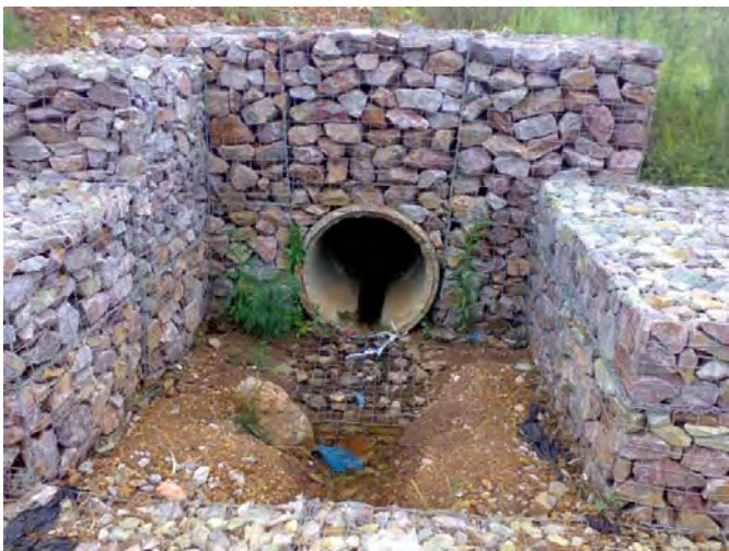
Design of the storm water outlets act as silt traps and litter traps. Vegetation will establish in outlets and gabions (2011)
