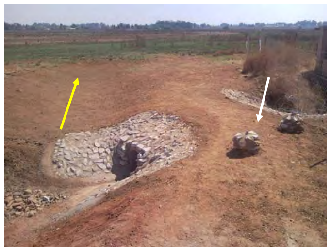
Revised design, with lower spillway for the 10yr or greater flood as well as barriers to restrict access to pan area (arrow)
