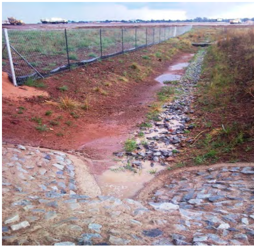
Bio-swale after rainfall – water pools within the bio-swale and creates new habitat (2010)
