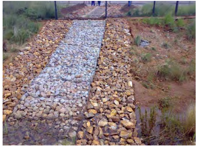
Additional rocks were placed on either side of the rock mattress to further minimize erosion in the bio-swale (2012)
