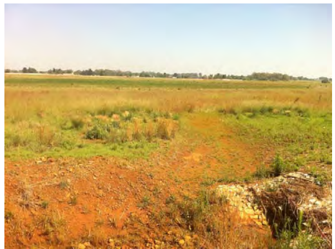
Spillway of the attenuation structure, as detailed above, shows the rehabilitation and progress of the spillways (2012)
