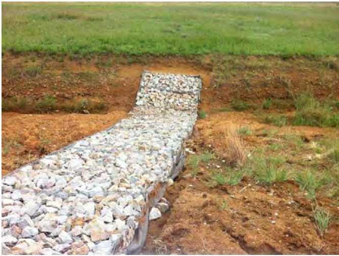
Commencement of storm water attenuation measures in the bio-swale to manage run-off from the Commercial site (2011)
