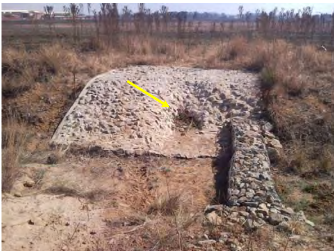
Low attenuation structures and gabions within the bio-swale. A subsoil drain was installed to feed the wetland (2010)
